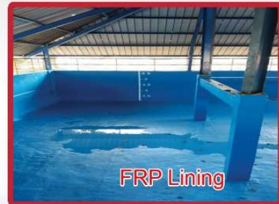
FRP Chemical Tank
